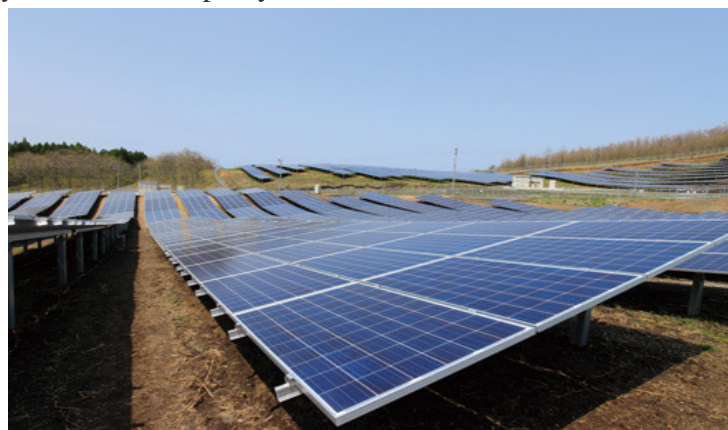
Figur 2 Kokonoe Solar Power Plant [4]
